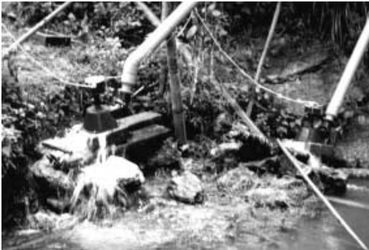
Figure 1 | "Sit-down" micro-hydroelectric systems
